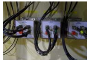
(c) SDA3EV1 amplifier
